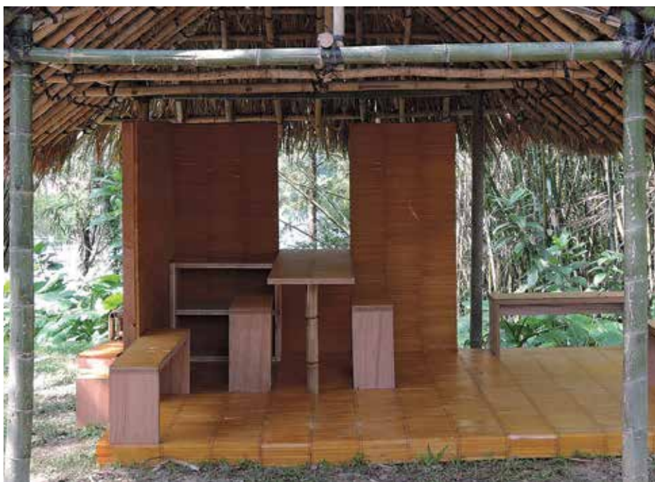
The hut is built by local scaffolding experts using vernacular construction and natural materials. Green bamboo poles form the primary structure, while reed especially cut from the Mai Po marshes are dried to form the roof's top layer, with the substantial thatch came from drying cut grass directly from the hills on campus. The walls, platform and furniture of the semi-interior setting are clad entirely using bamboo scrolls to embody the scholarly ambience.
